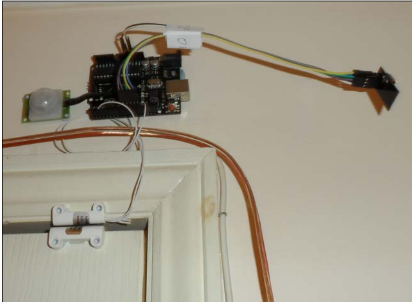
The sensor node with a door switch and PIR sensor installed above a door frame using Blu-Tack
